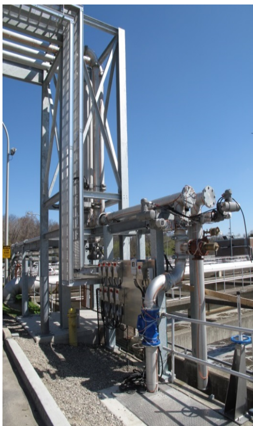
Unique supply infrastructure associated with SOWC's London Wastewater Facility
